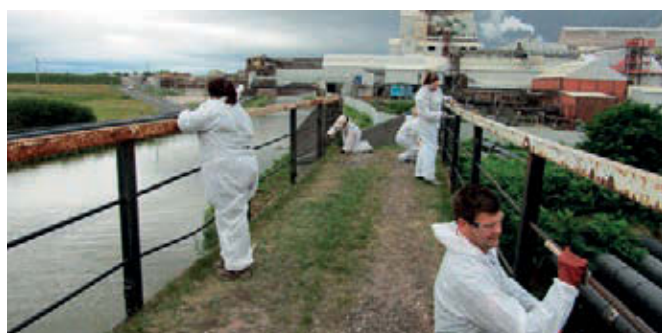
Head Office team volunteered their time on the Northwich section of the Trent and Mersey canal
